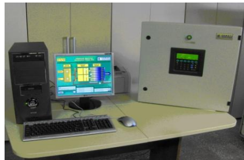
Wastewater Treatment Plant Monitoring and Control
