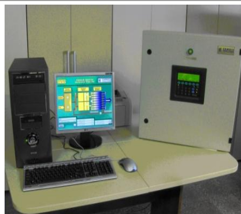
Wastewater Treatment Plant Monitoring and Control
