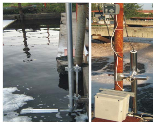
Control of the dissolved oxygen concentration in a wastewater treatment plant
